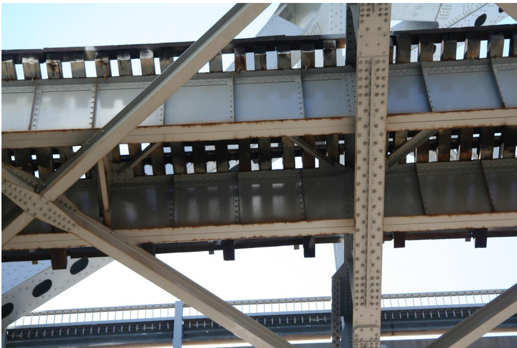
Condition Photo 18: Underside of railroad portion of east approach spans; shows bolted strengthening of floor beam bottom flange.
