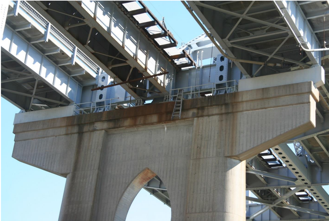
Condition Photo 9: Pier 1 and three approach spans supported on pier; beginning of truss span, looking at eastbound roadway.
