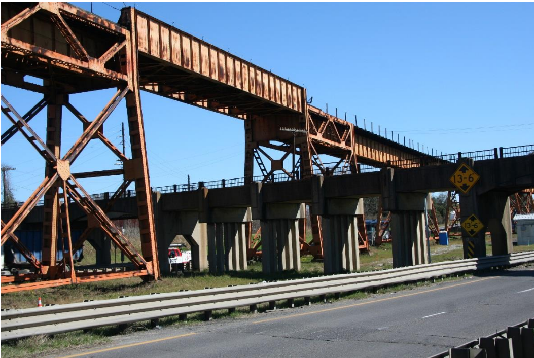
Condition Photo 28: Railroad easterly approach spans over the CNRR, to be painted in 2016, looking east. Note vertical clearance sign for eastbound US 190 under the CNRR bridge.
