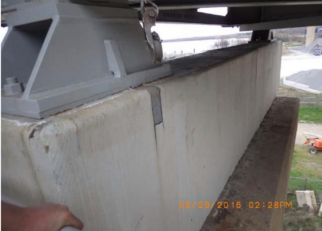
Condition Photo 23: View of fiber wrap failing on pier 1 north side. (Photo courtesy of LADOTD from March 3, 2016, inspection report.)
