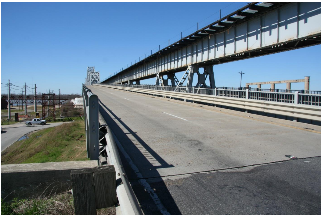
Condition Photo 20: Eastbound roadway at east abutment; note bridge deck expansion joint and approach road pavement condition.
