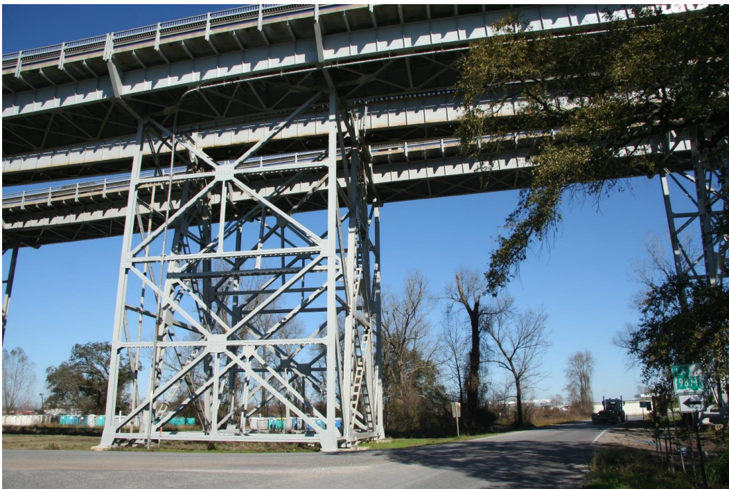
Condition Photo 8: Steel tower bent and approach spans at River Road.
