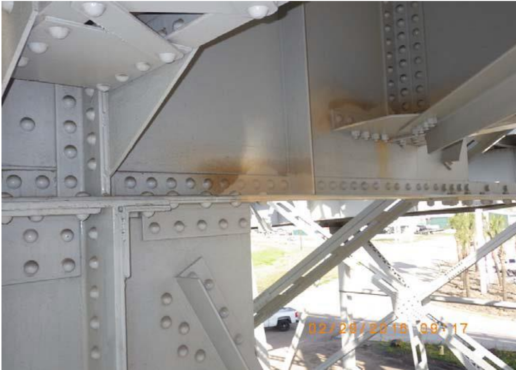
Condition Photo 21: View of typical minor rust stains to floorbeams and steel members found throughout the structure. (Photo courtesy of LADOTD from March 3, 2016, inspection report.)
