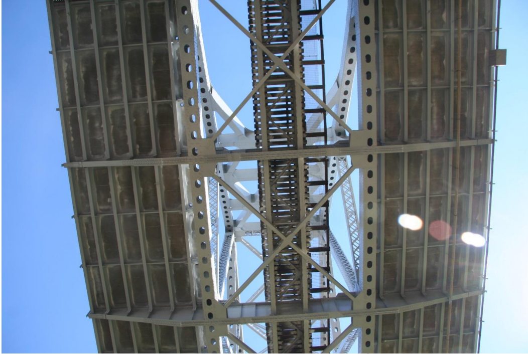
Condition Photo 11: Underside of truss span 1; railroad in middle, highway on each side.
