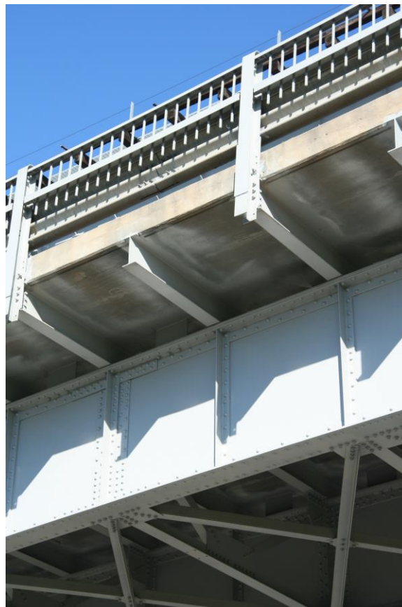
Condition Photo 4: South side of steel girder approach span, showing widened roadway deck and bridge railing details including attachment.
