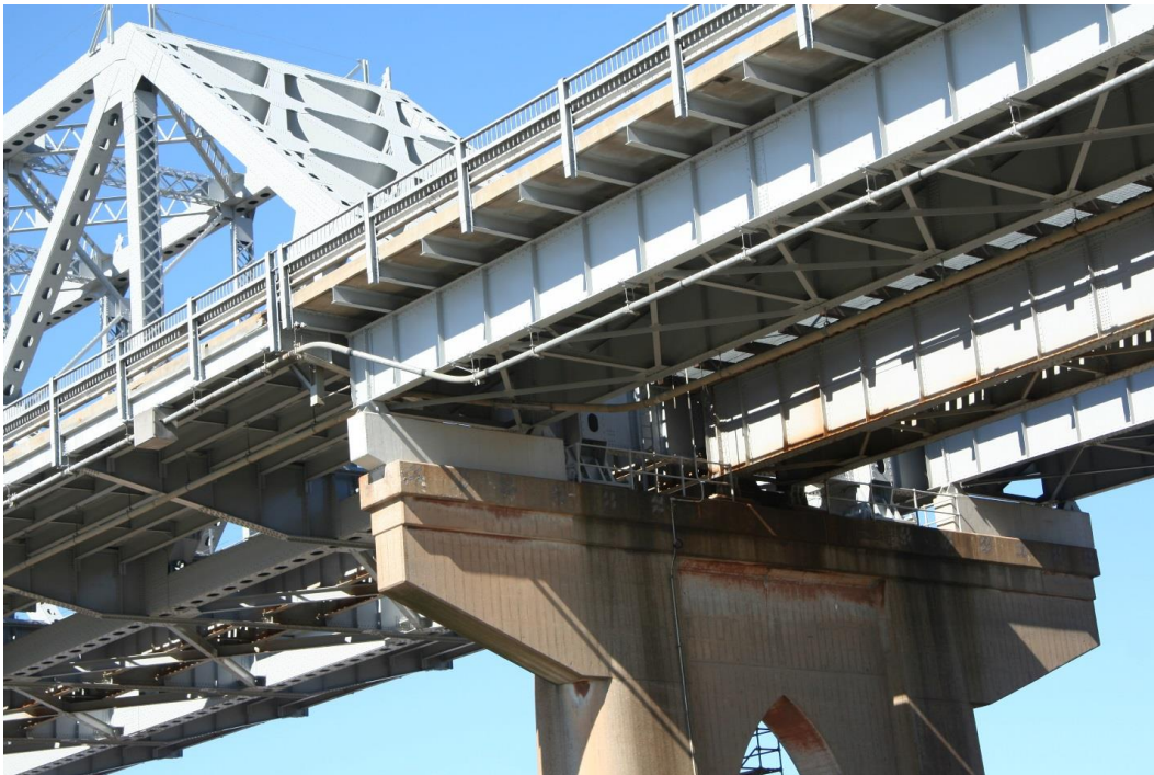
Condition Photo 16: Pier 6 and approach spans supported on pier; beginning of truss span, looking at eastbound roadway.
