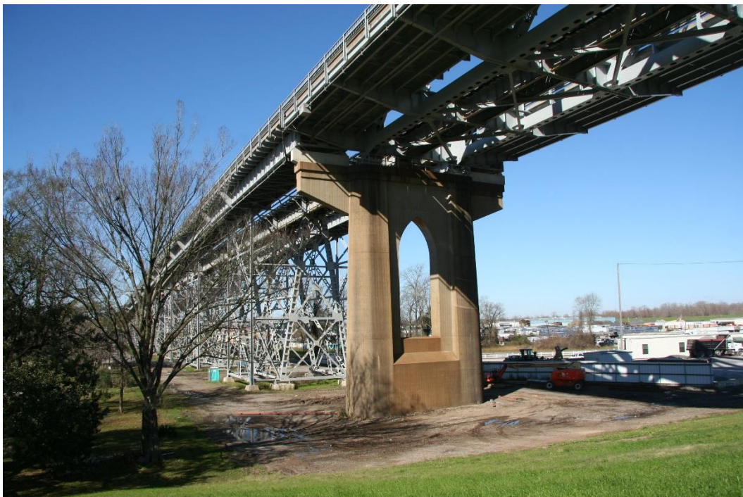
Historic Fabric Photo 4: Piers and braced steel columns comprise substructure elements on the western approach spans of the bridge.
