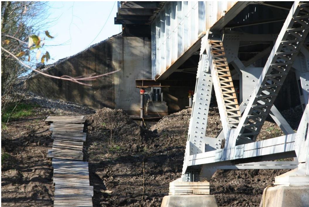
Condition Photo 26: Bearing rehabilitation at west abutment of railroad west approach spans.
