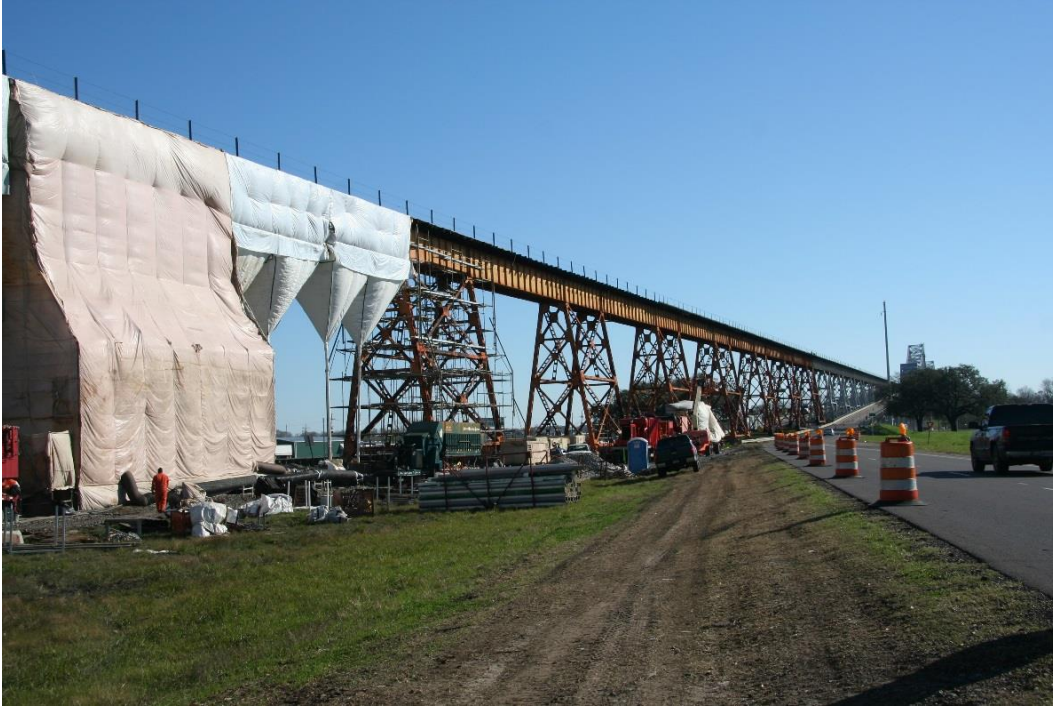
Condition Photo 27: Railroad westerly approach spans, cleaning and painting with containment system, looking east (as of February 2016 site visit).
