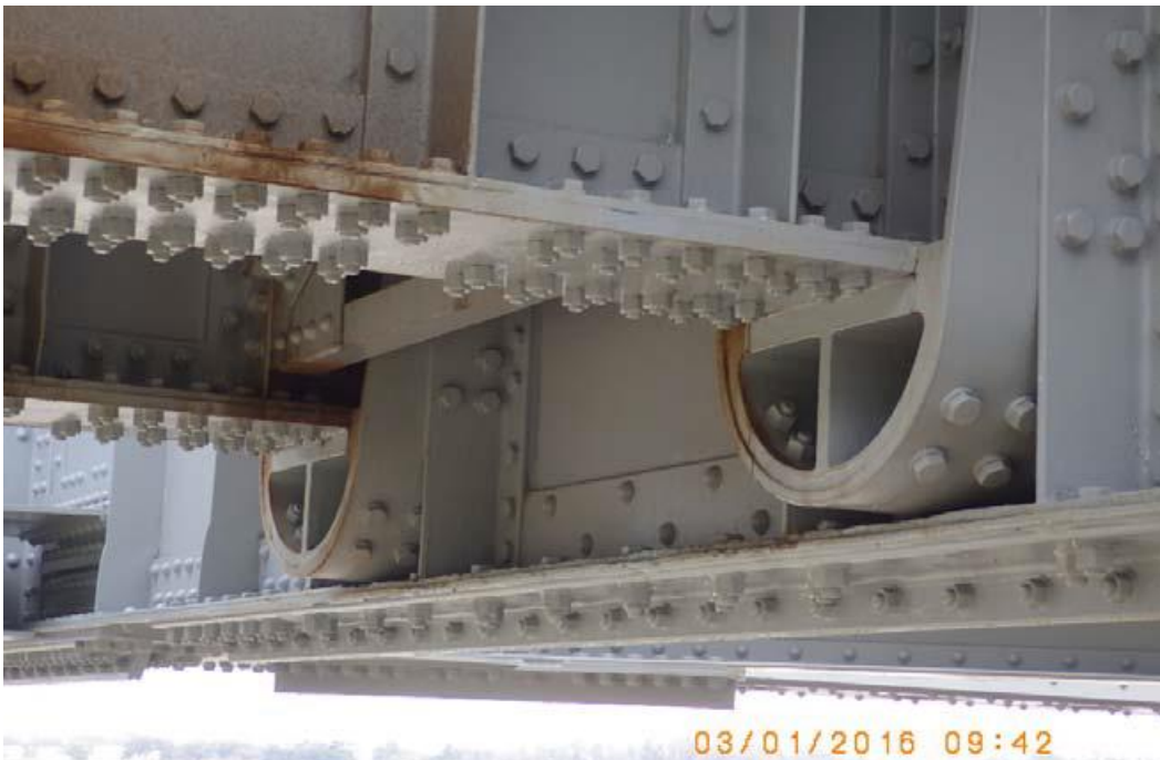
Condition Photo 22: View of typical minor rust stains to girders at saddle bearings found throughout the structure. (Photo courtesy of LADOTD from March 3, 2016, inspection report.)
