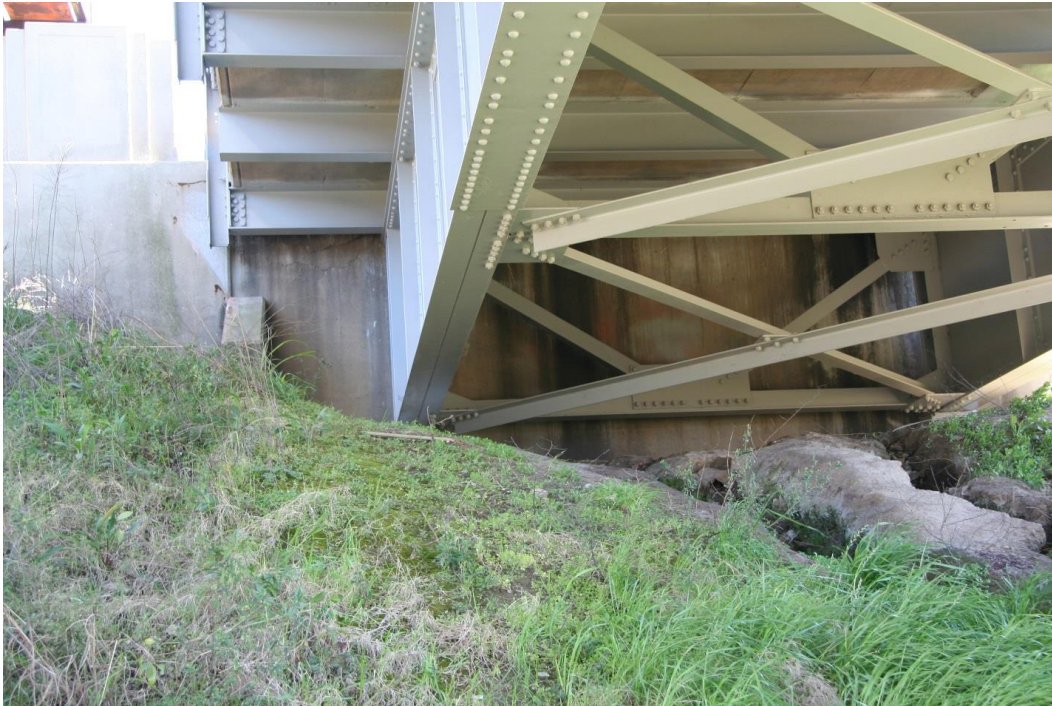
Condition Photo 19: Eastbound roadway east abutment showing erosion under bridge.
