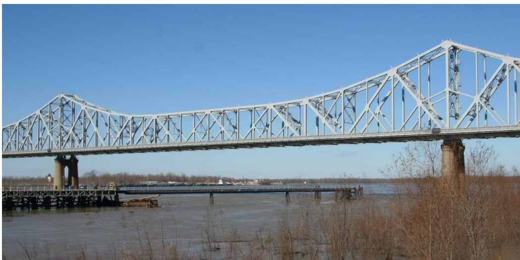
Character-defining Feature Photo 2: Cantilevered design to carry both railroad and vehicular traffic by suspending the roadways laterally from both sides of the truss spans.
