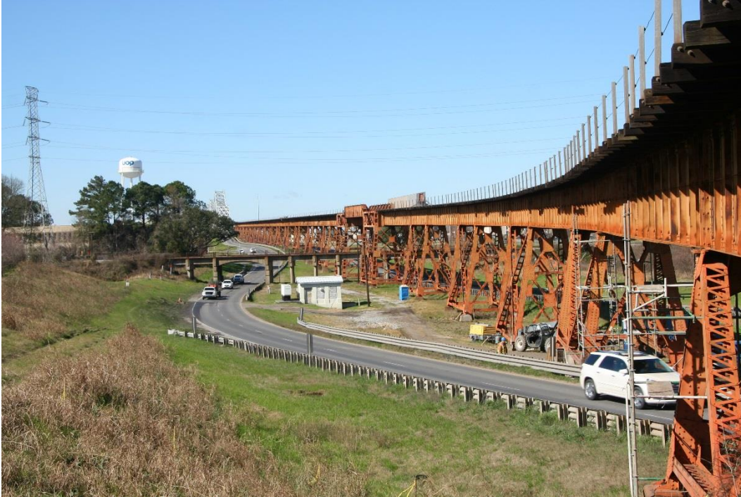
Condition Photo 29: Railroad easterly approach spans to be painted in 2016, looking west.
