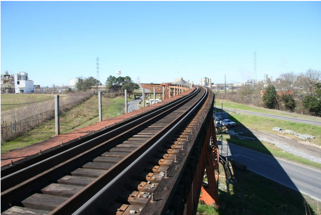
Condition Photo 30: Railroad east approach spans deck, looking west; walkway to be removed and replaced in 2016 with a metal grating walkway with cable handrail.
