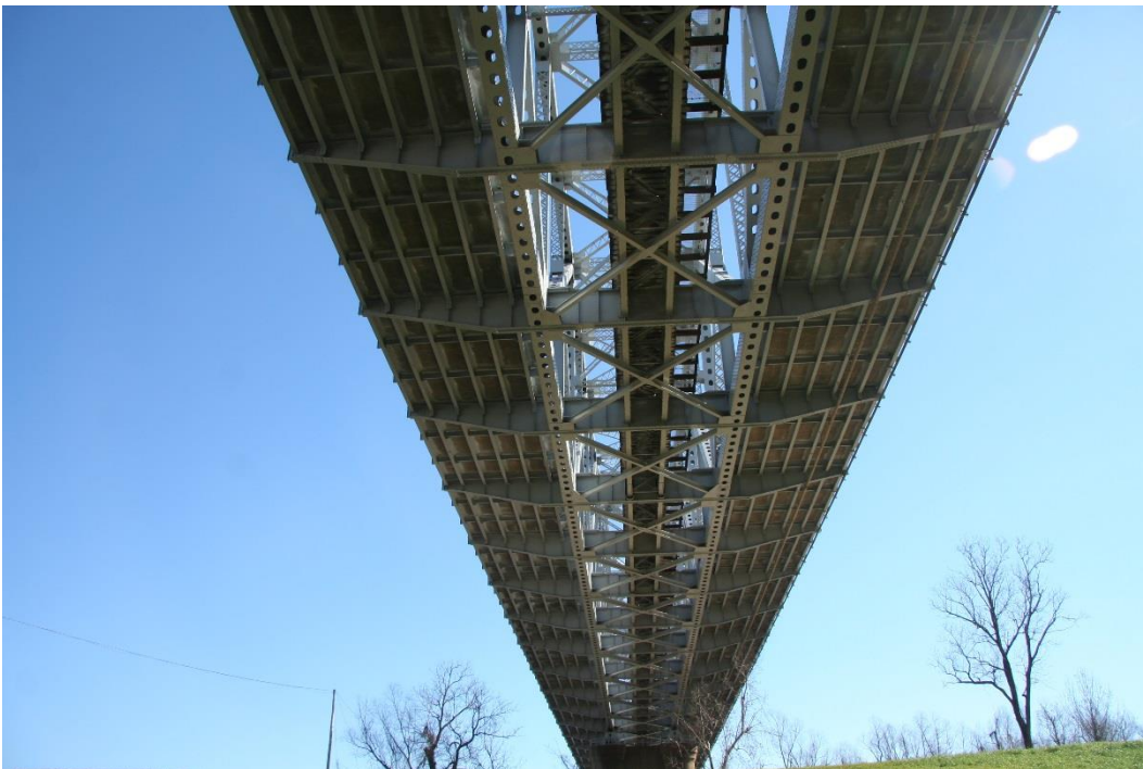
Historic Fabric Photo 2: Original materials of the floor system under the truss spans.
